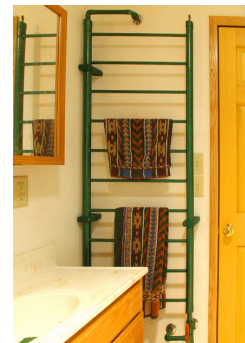
Fig. 14: Hydronically heated towel rack
