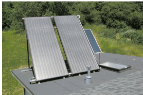
Fig. 4: Solar thermal panels and PV power for pump
